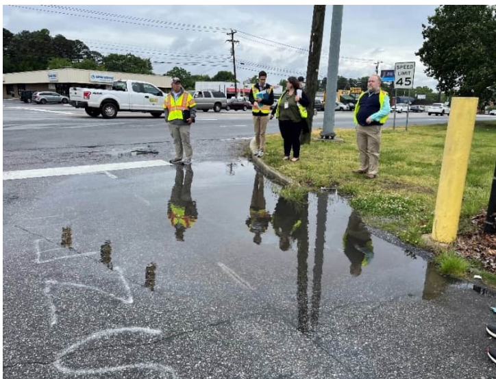
Drainage issues on westbound approach of intersection
